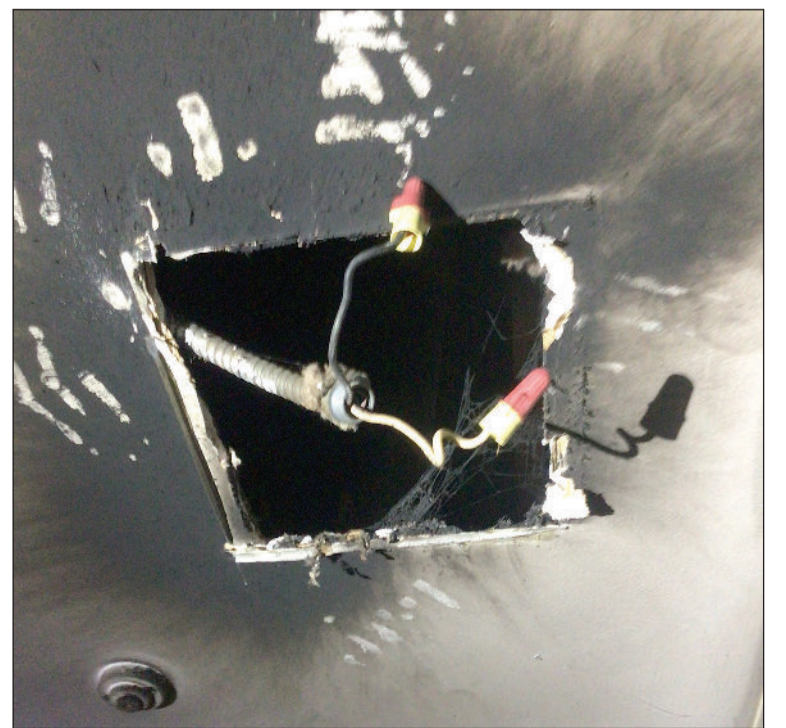
Damage to the ceiling in a restroom at Dublin Trails/SPECIAL PHOTO
