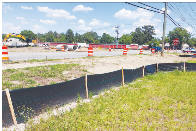
Work on the new roundabout at Woodlawn Drive and Claxton Dairy Road has already begun. The intersection will be closed to traffic beginning Tuesday/PAYTON TOWNS III
