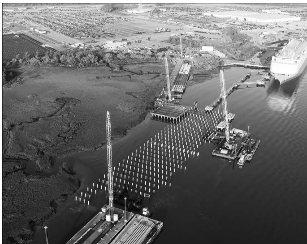
A fourth berth under construction at the Port of Brunswick's Colonel's Island will handle a mix of autos, heavy equipment and project cargo. The new dock will go into service in 2027/SPECIAL PHOTO, Georgia Ports
