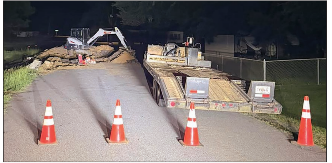
Crews worked on the water main break into the early hours of Thursday morning/SPECIAL PHOTO, City of Dudley
