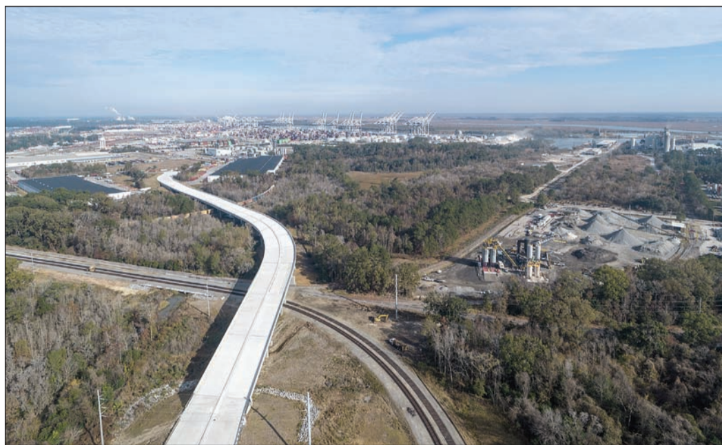
The $126 million Brampton Road Connector links the Port of Savannah's Garden City Terminal to the Interstate 16 corridor/SPECIAL PHOTO, Georgia Ports Authority
