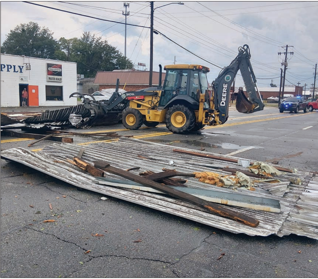
A backhoe cleans up a roof and other debris from Cullens Supply & Engine Services after Sunday afternoon's storm/SPECIAL PHOTO, Dublin Fire Department
